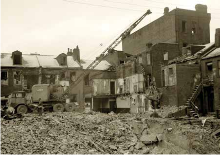
Buildings being razed in the Lower Hill District as part of Pittsburgh's renaissance and urban renewal programs, January 2, 1957.
